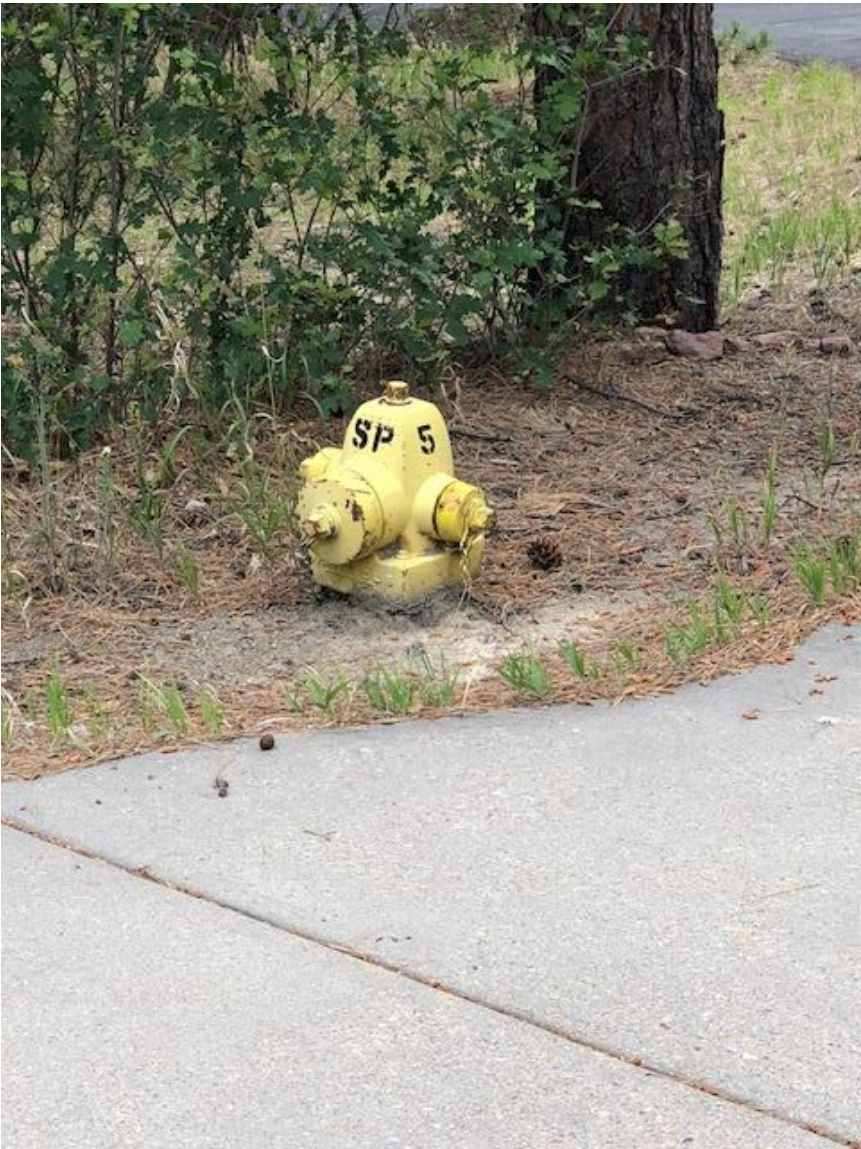
Fire Hydrant 17180 Oxbridge Dr.
